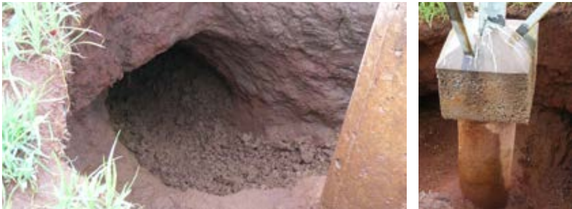
Porcupines burrowed at the base of the transmission towers along the Matla/Benburg line. Photo credit: Constant Hoogstad
