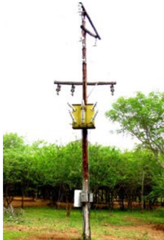
Transformer in Marloth Park. Photo credit: Marloth Park
