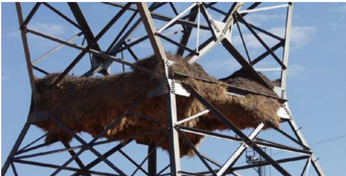
Sociable Weaver nest on a transmission tower. Photo credit: Jon Smallie
