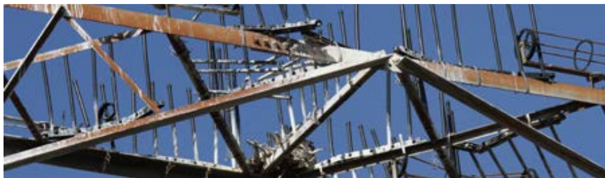
Reed Cormorants polluting insulators while nesting or roosting on a transmission line. Photo credit: Matt Pretorius
