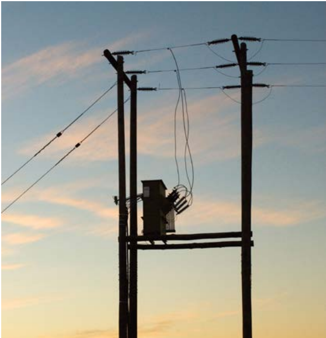
Insulated box transformer. Photo credit: Marianne Golding
