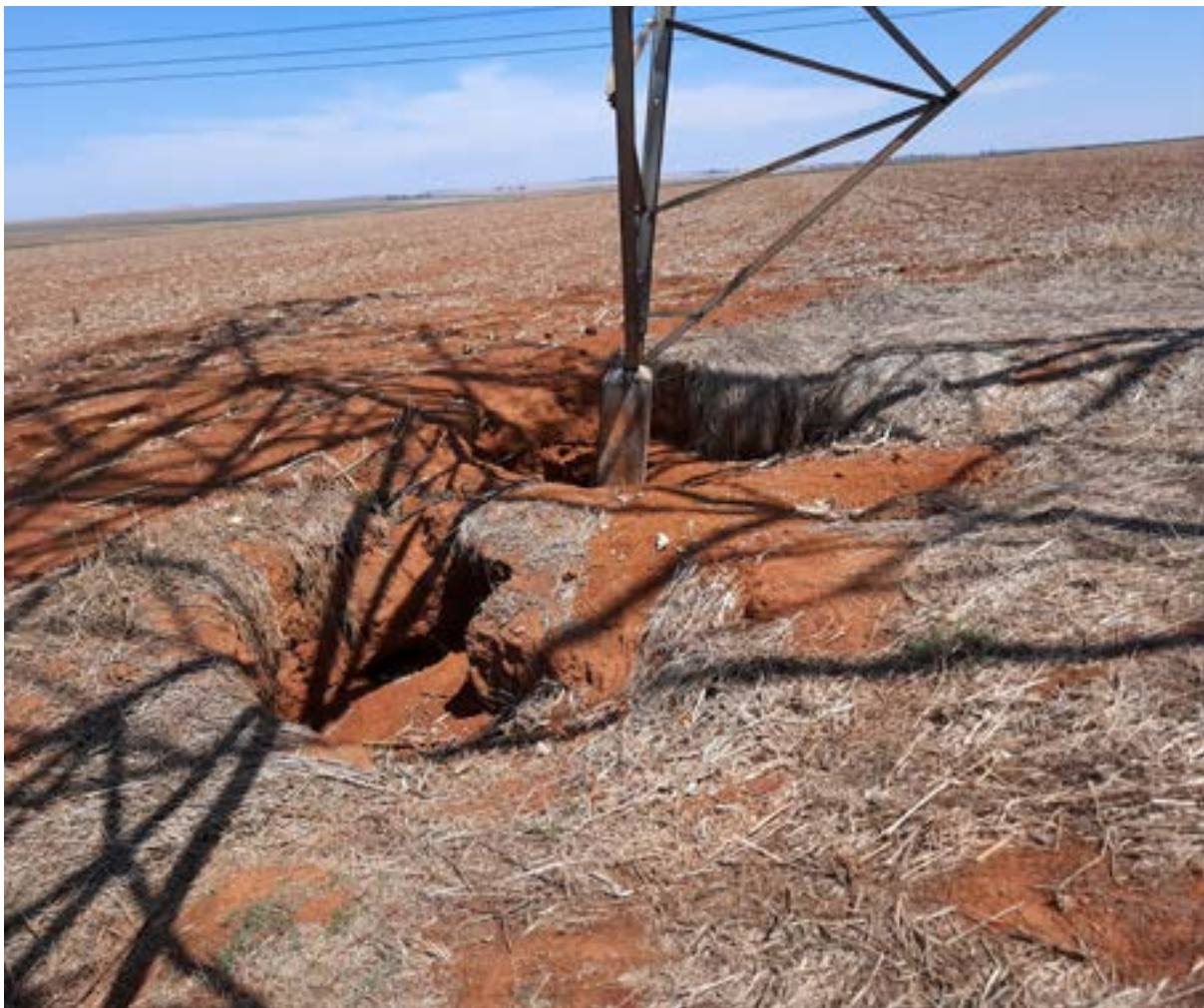
Porcupine excavations around a lattice tower foundation. Photo credit: Ndzalama Chauke
