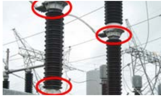
Flash marks shown on hardware inside the substation where the python was electrocuted.
